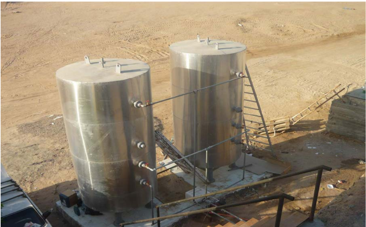
2 * 5 m 2 Solar Tank
