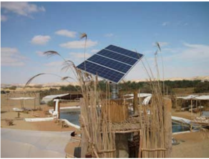
PV system for Pool Circulation
