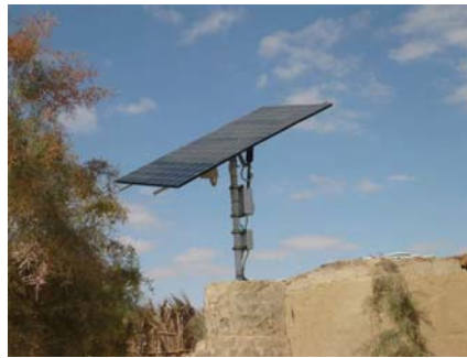
PV system for Submersible Solar Pumping
