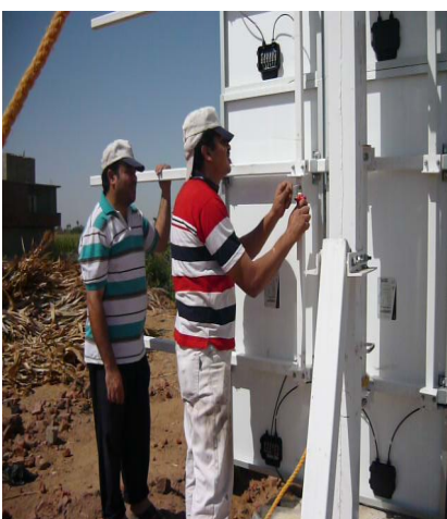
PV Cable Connection
